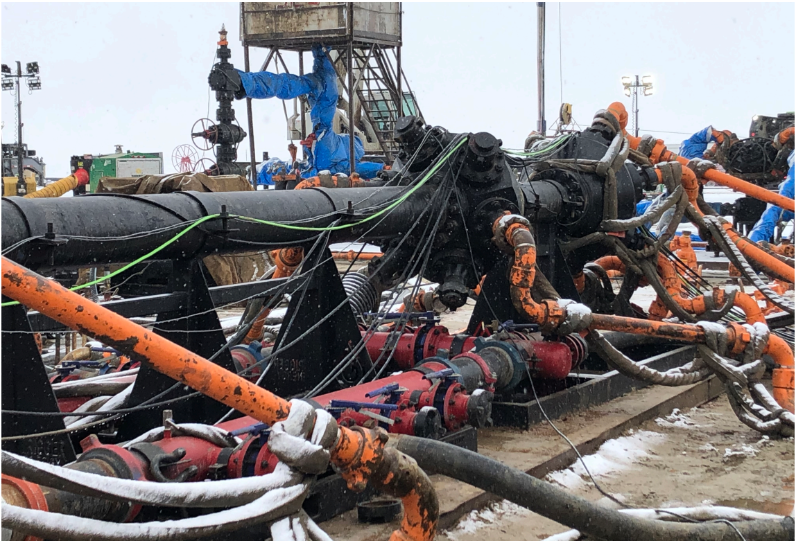
Figure D. 2 - Monoline with low and high pressure circuits. Photograph taken in Wyoming.
