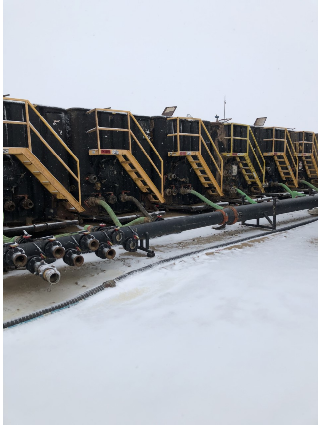
Figure D. 1 - Static water tanks holding fluid to be used for stimulation. Photograph was taken in Wyoming.
