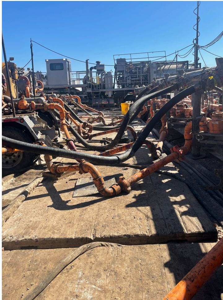
Figure D. 3 - Frac pumps hooking up to missile, converting low pressure fluid to STP. Photograph was taken in North Dakota.
