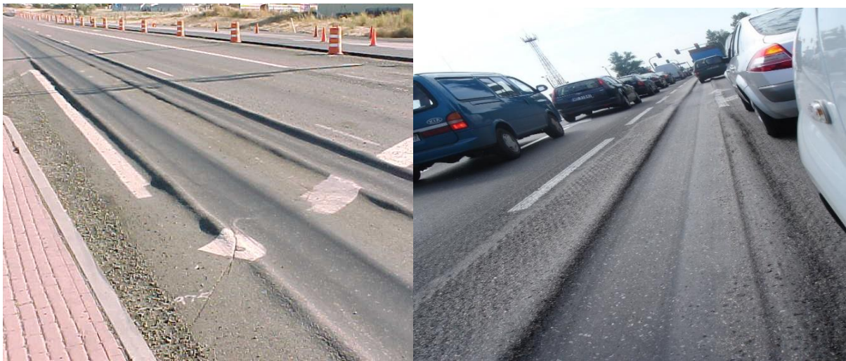
Figure 2.1 Rutting Distress in Asphalt Pavements (Wang et al., 2021).
