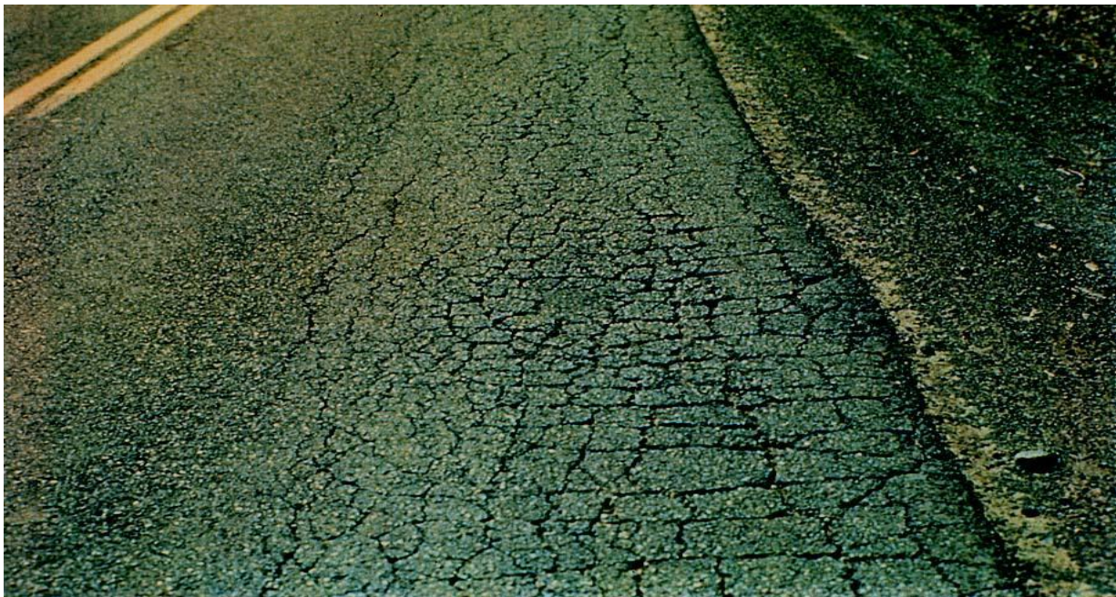
Figure 2.3 Fatigue Cracking (Alligator Cracking) in Asphalt Pavements (Wang et al., 2021).
