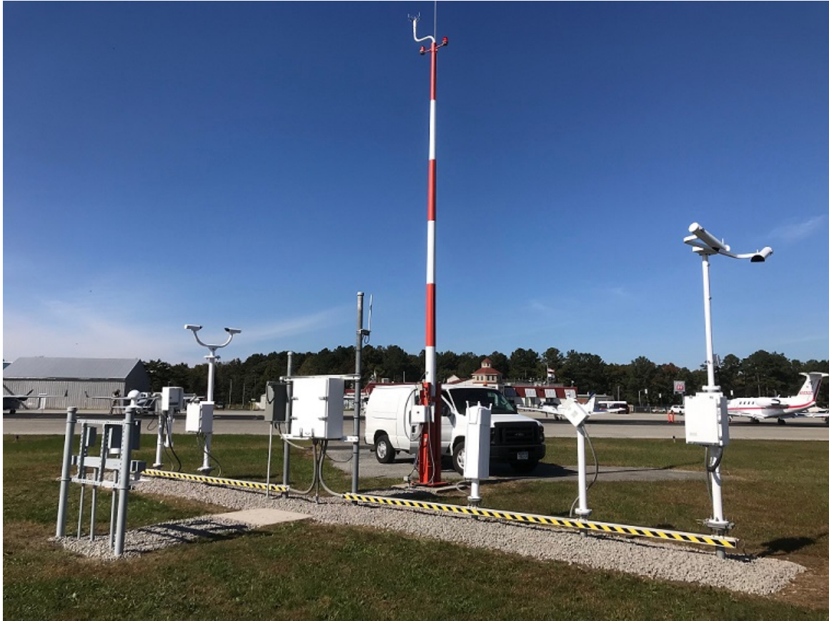
Figure 7. Example of an Automated Surface Observing Station (ASOS Users Guide 1988).
