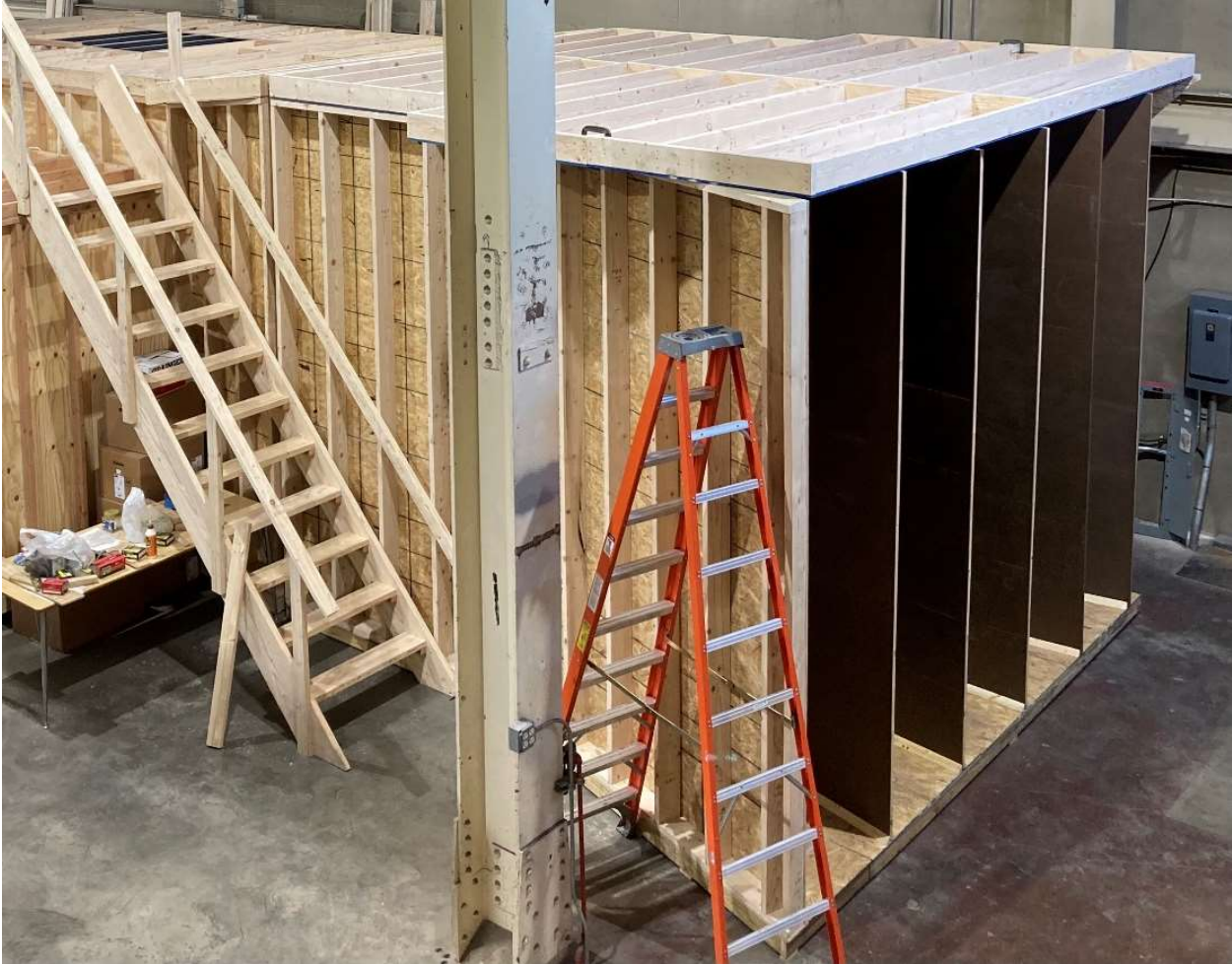
Figure 29. Constructed Multi-vane Diffuser Rear View
