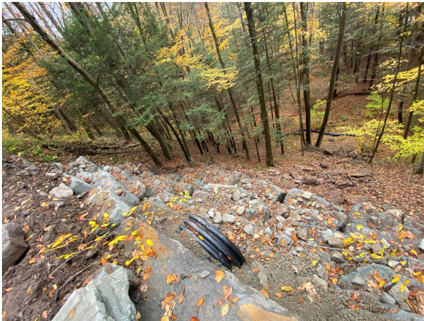
Image 3: View of rockery wall and drainage pipe from top of road, directly above rockery wall at Site 1 at Worlds End State Park
