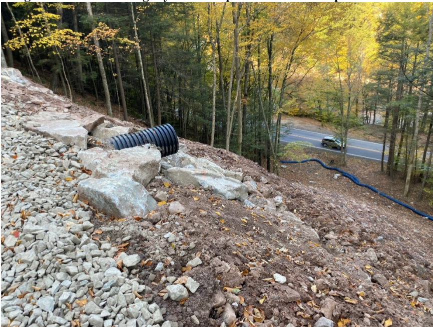
Image 6: View of drainage system at top of remediated slope at Site 2 at Worlds End State Park
