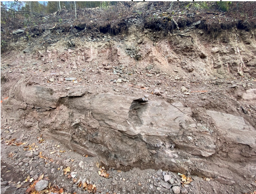
Image 9: View of sandstone at base of proposed steep slope at Loyalsock State Forest
