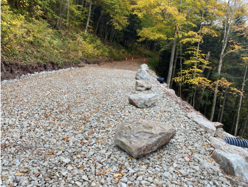
Image 5: View of roadway grade above remediated slope at Site 2 at Worlds End State Park
