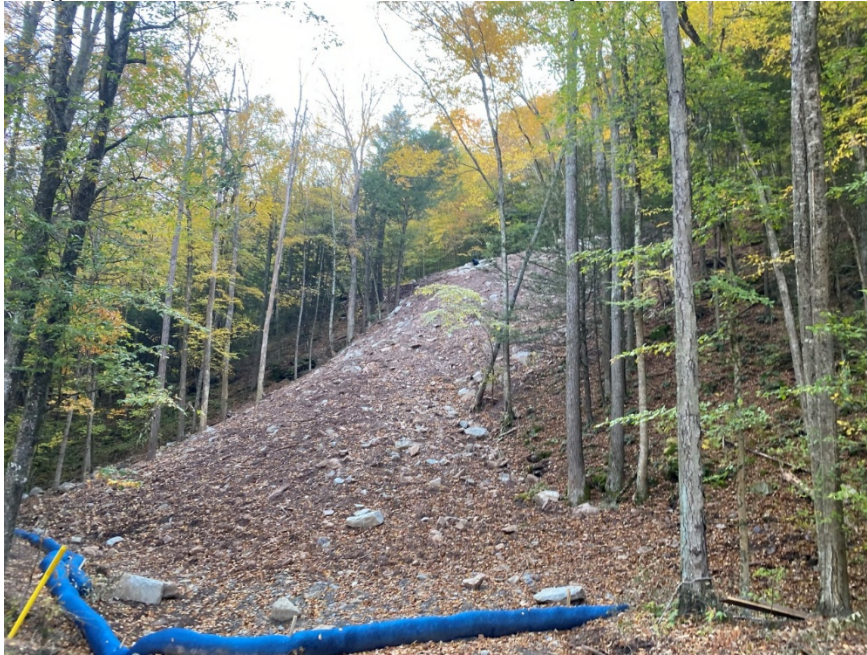
Image 7: View of remediated area from down-slope at Site 2 at Worlds End State Park
