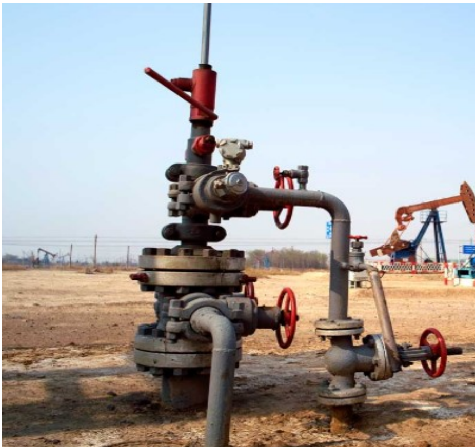
Figure 1. Wellhead from primary production
