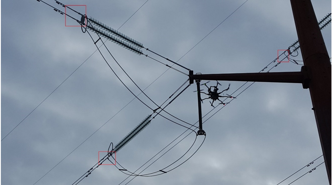
Figure 2: Image of UAS collecting DEBC inspection images. Regions in red contain DEBCs.
