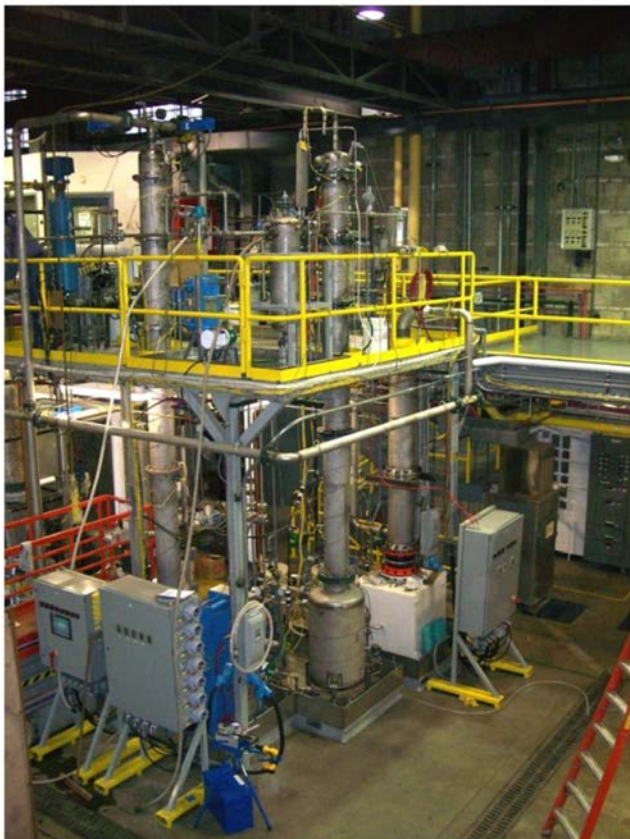
Figure 15. SASC system as tested during shakedown.
