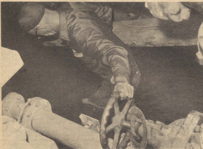
Al Marsh, Buildings and Grounds crew member, helped with repairs on the swimming pool.
