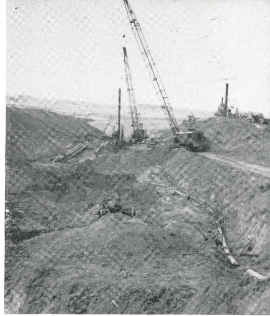
SHEETPILE WALL IS DRIVEN in sections in core trench excavation on right bank where necessary to cut off deeper pervious strata. Maximum sheetpiling length of 50 ft used here does not require tower for driving.
