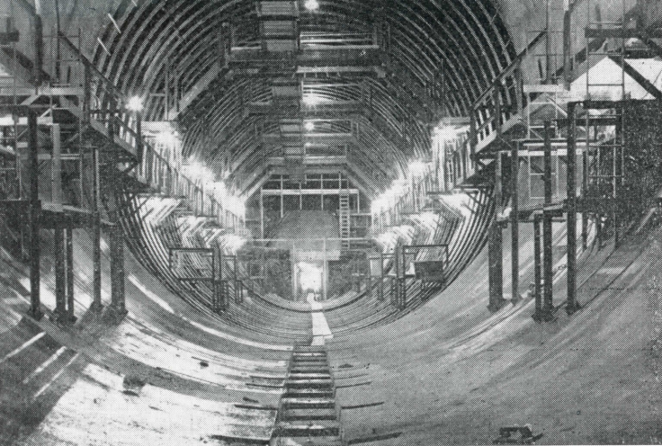
TEST TUNNEL (left) completed in January 1949, at site of penstock tunnel No. 4, contains instruments to record magnitude and distribution of earth pressures. Catwalks give access to instruments and measurement points. Slots in concrete lining at invert expose sections of steel ribs for strain-gage measurements.
