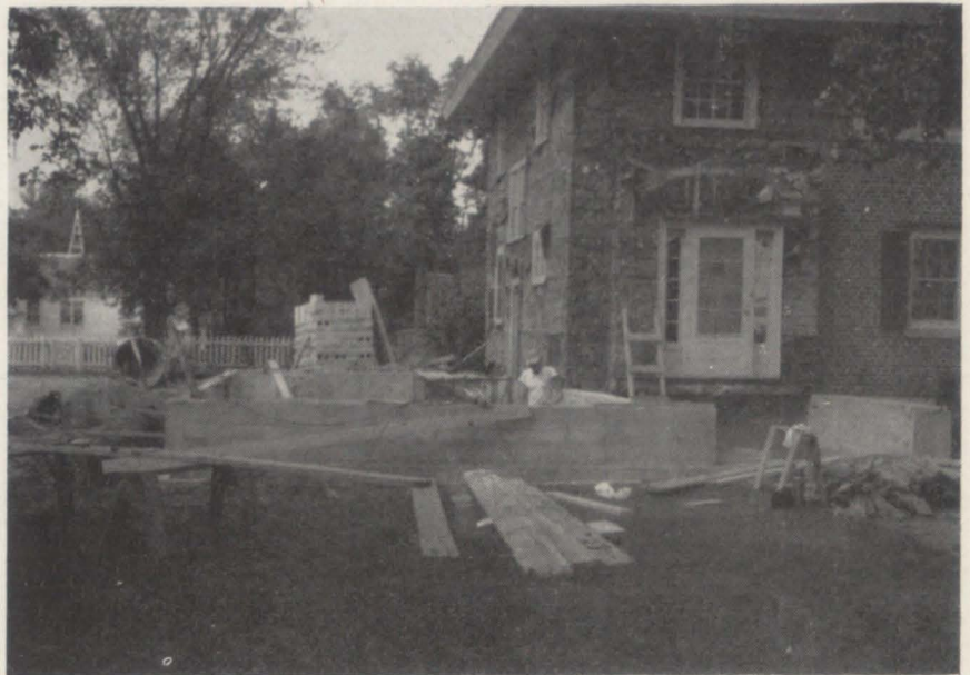
Progress is being made on the addition to the Kappa Alpha Theta sorority house at 2500 University Avenue. The addition will provide a new dining room and expansion of the kitchen, as well as seven new bedrooms. The Theta's also are expanding their living room into the area previously used for dining and are redecorating the third floor bedrooms.
