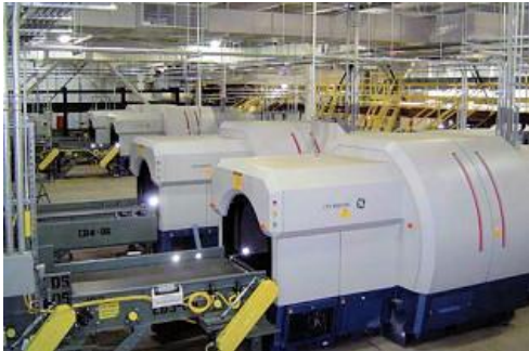
Figure 3. Airport Inline Screening System
