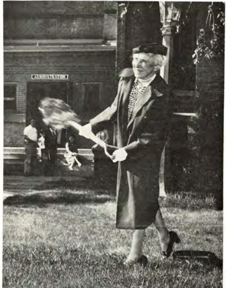
Miss Edna Twamley breaks ground for Twamley Hall, new UND administration building.
