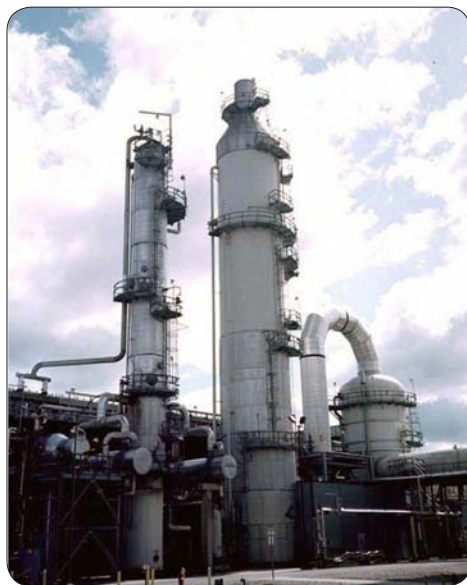
Fluor's Econamine FG SM plant at Florida Power and Light's facility located at Bellingham, Massachusetts (Reddy et al., 2008). The Econamine FG plant has a capacity of 330 tons/day of food-grade CO 2 or 300 to more than 3000 times smaller than a power plant.
