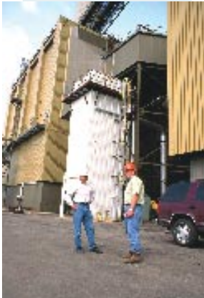
During a successful demonstration of the advanced hybrid particulate collector (AHPC) at Otter Tail's Big Stone power plant, EERC Senior Research Manager Stan Miller, left, visited with Bill Swanson, an engineer at the plant.
