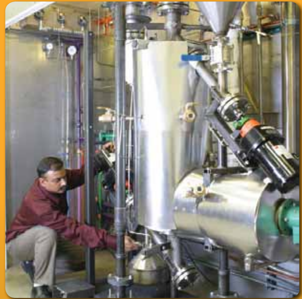
The EERC is integrating biomass gasification with state-of-the-art solid oxide fuel cell technology.
