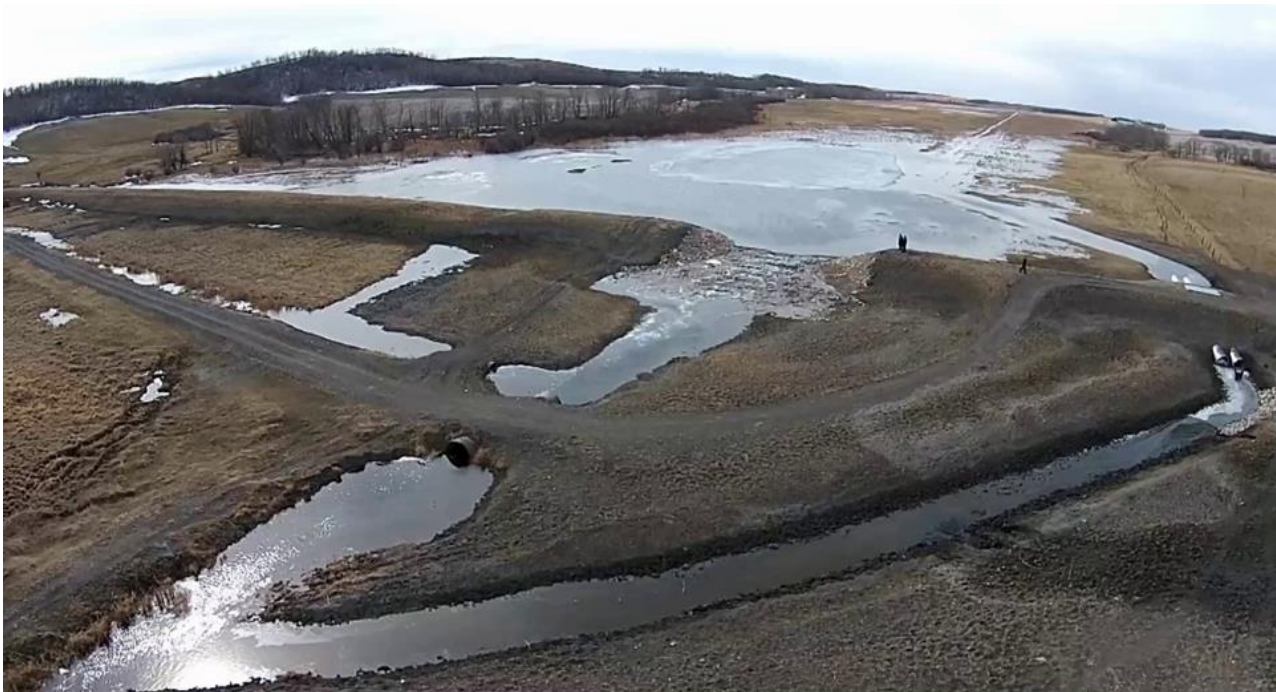
Figure 2. Aerial view of the Pelly's Lake Water Management Project in operation retaining spring runoff water (20 March 2015). Wetland habitat extends to the horizon, areas of harvested cattail in the deepest section closest to the earthen dam is fully under water. Opening of the gated culverts (right side of photo) will lower water levels allowing new wetland habitat to emerge. The ability to control water levels allows for autumn harvest of biomass.
