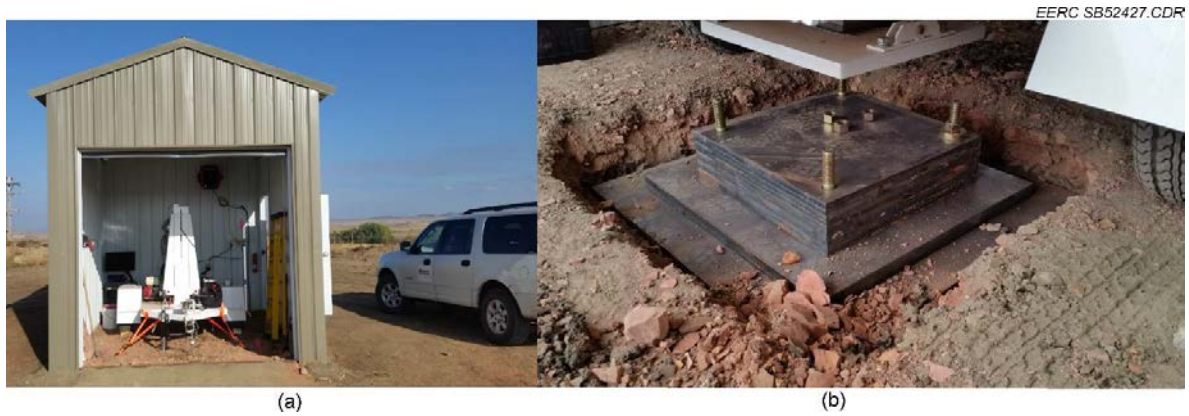
Fig. 4. (a) Completed shed wired for power showing the installed and anchored ESS850 source, remote control computer system (back left corner), and space heater (mounted on rear wall). (b) Engineered footing shown during assembly and before burial. The footing is dug in to place the top plate at grade. The coupling plate on the ESS850 is removed so that the hammer directly strikes the footing [10].
