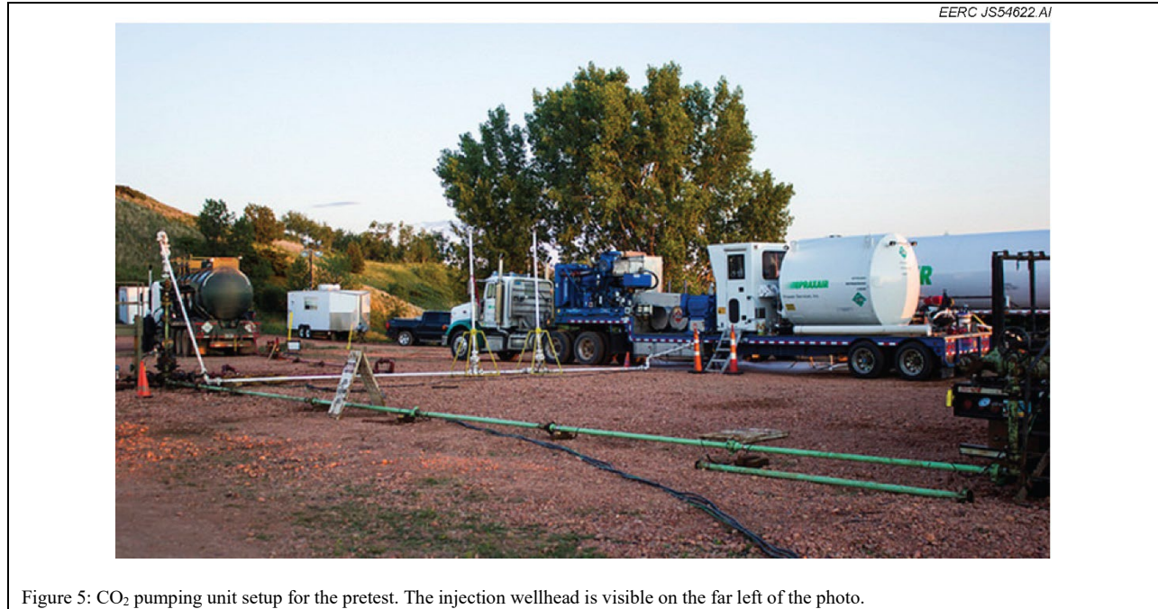
Figure 5: CO 2 pumping unit setup for the pretest. The injection wellhead is visible on the far left of the photo.
