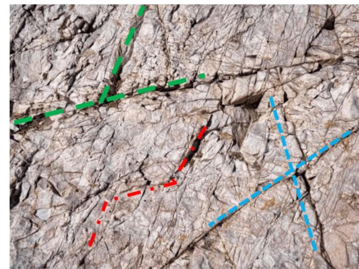
Fig. 1. Fractures in a rock outcrop highlighting the most common naturally occurring: the blue is the X-crossing fracture, in red the Z fracture, and green is the Y fracture
